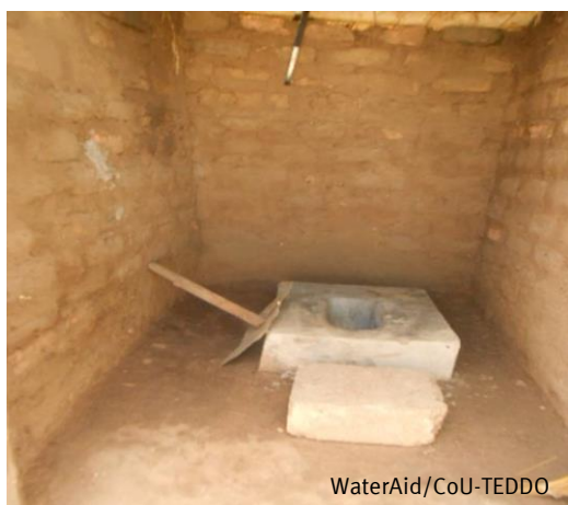
A raised fixed latrine seat made out of cement.
