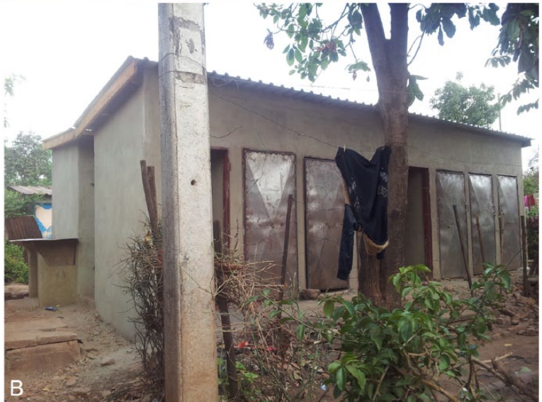
PHOTOS 2A AND 2B Sanitation block in Gadzema before and during construction
